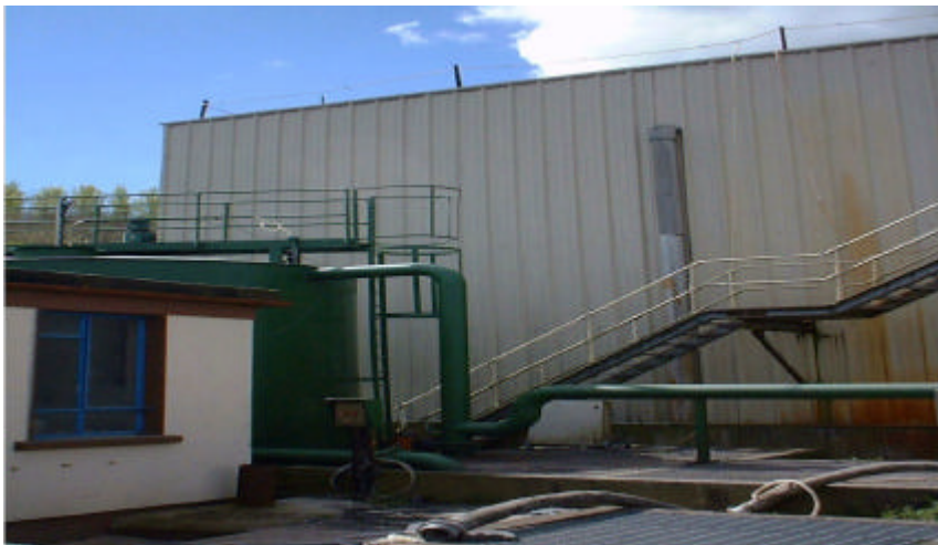
View of the Bio-tower in Dairygold.
